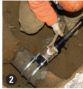
2 Open corp stop valve.
